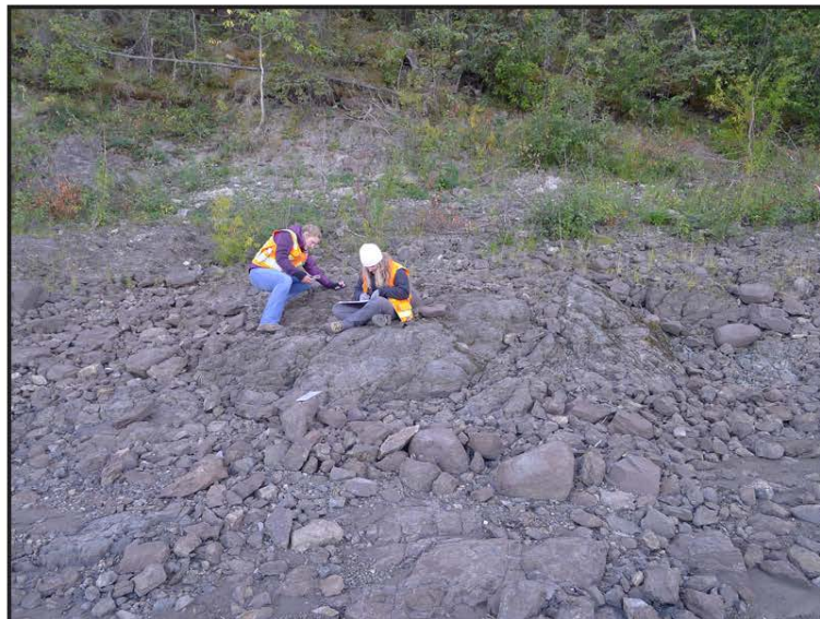
A11. Station 9 joint sets, between 100 and 150 feet east of the Yukon River bridge.
