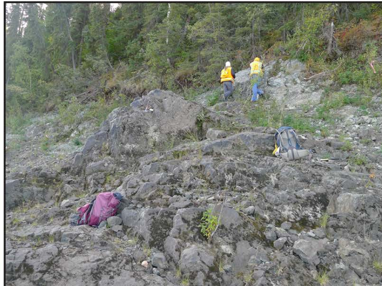
A5. Station 4b joint sets, 250 feet west of the Yukon River bridge and east of the landslide.
