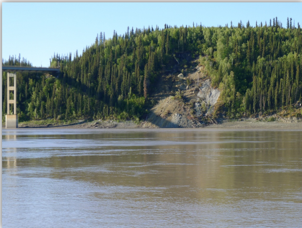
Yukon River bridge landslide viewed from the north bank of the Yukon River. Photo by Rich D. Koehler
