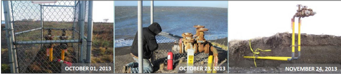
Figure 13. Fuel header pipes for Port Heiden's bulk fuel farm undercut by the eroding bluff during the 2013 storm season (photos by Linda Anderson, LEO).
